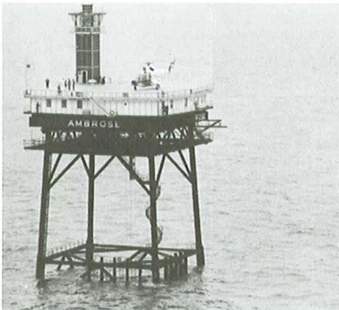
The Ambrose Offshore Light Tower, 7 miles east of Sandy Hook, New Jersey. Its primary light has a high intensity of 6 million candlepower with a charted range of 18 miles.
